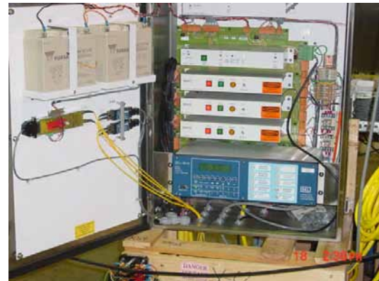
Figure 4—Each switchgear package is equipped with fiber-optic modem/transceiver, current and voltage sensing equipment, and an SEL-351S Protection and Breaker Control Relay.
