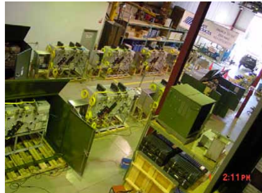
Figure 6—Acceptance testing of the Lake Pontchartrain Causeway power system control is shown above at the Canada Power Products factory.
