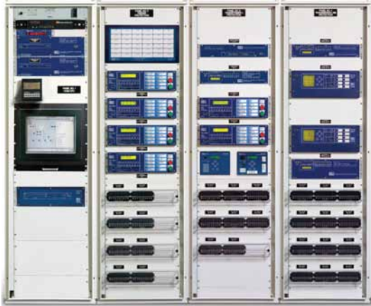
Figure 3—The SEL-7000 Integrated Substation System was installed in a separate communications panel containing communications equipment and the HMI system.
